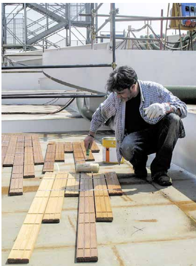
Fig. 9 Applying Sika® Primer-290 DC or Sika® MultiPrimer Marine to a teak deck with a roller (hidden side)
